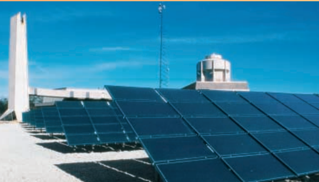
A grid-connected photovoltaic array at Alliant Energy in Winnebago, Minnesota. It can be used to bridge any supply shortfalls at peak times.
