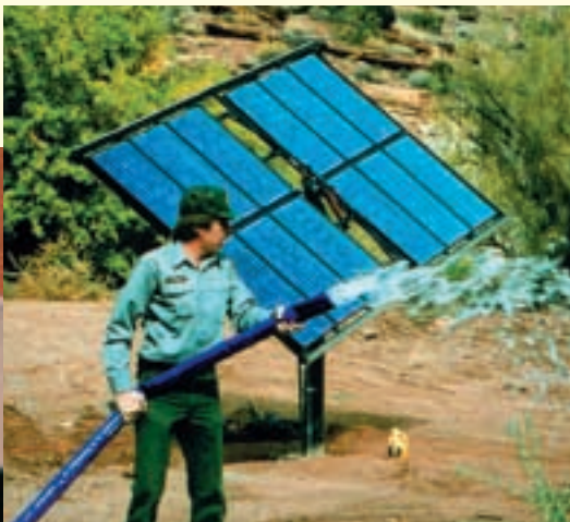
An environmentally friendly alternative to diesel generators: The Capitol Reef National Park in Utah uses photovoltaic modules to pump water from deep below ground.
