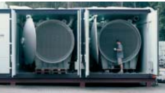
The ozone generators are installed in large-capacity containers.
